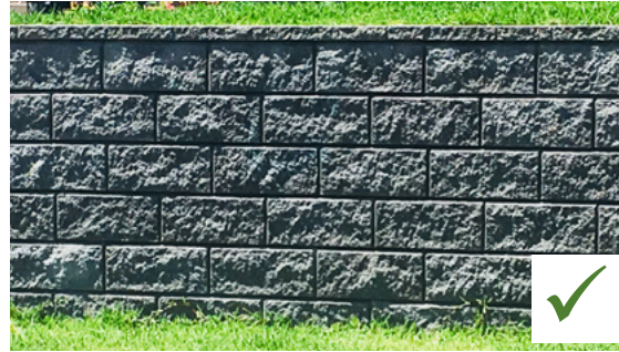
RETAINING WALLS – to be constructed from masonry or natural stone whenever visible from the street. Dark grey or charcoal colour preferred.
